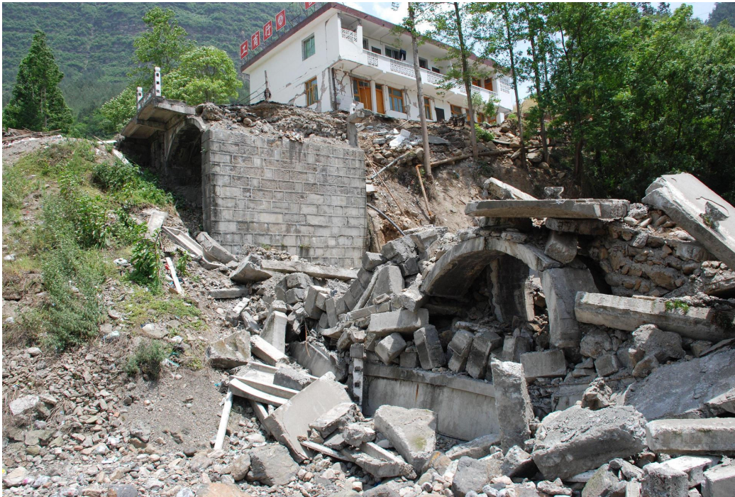
Collapsed arch bridge
